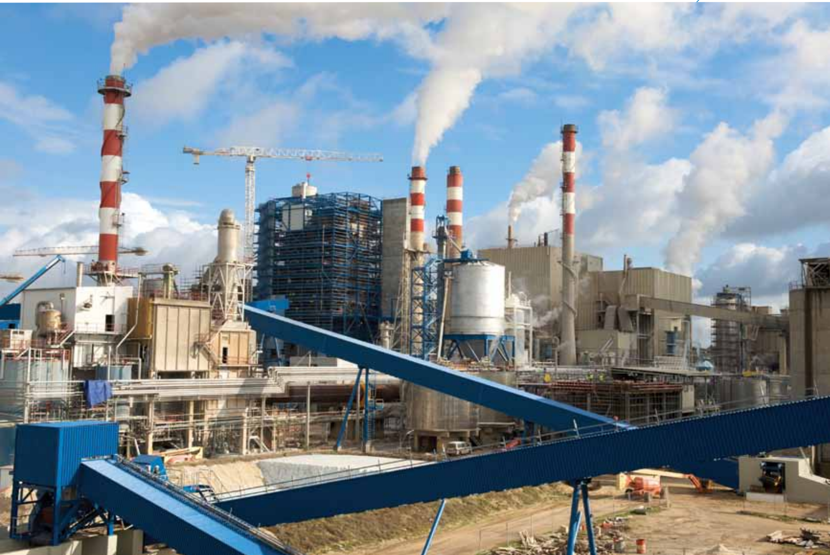
2008 / FIGUEIRA DA FOZ - PORTUGAL Prefabrication and Erection of Piping, Equipment and Steel Structures for CELBI (Paper Plant)
