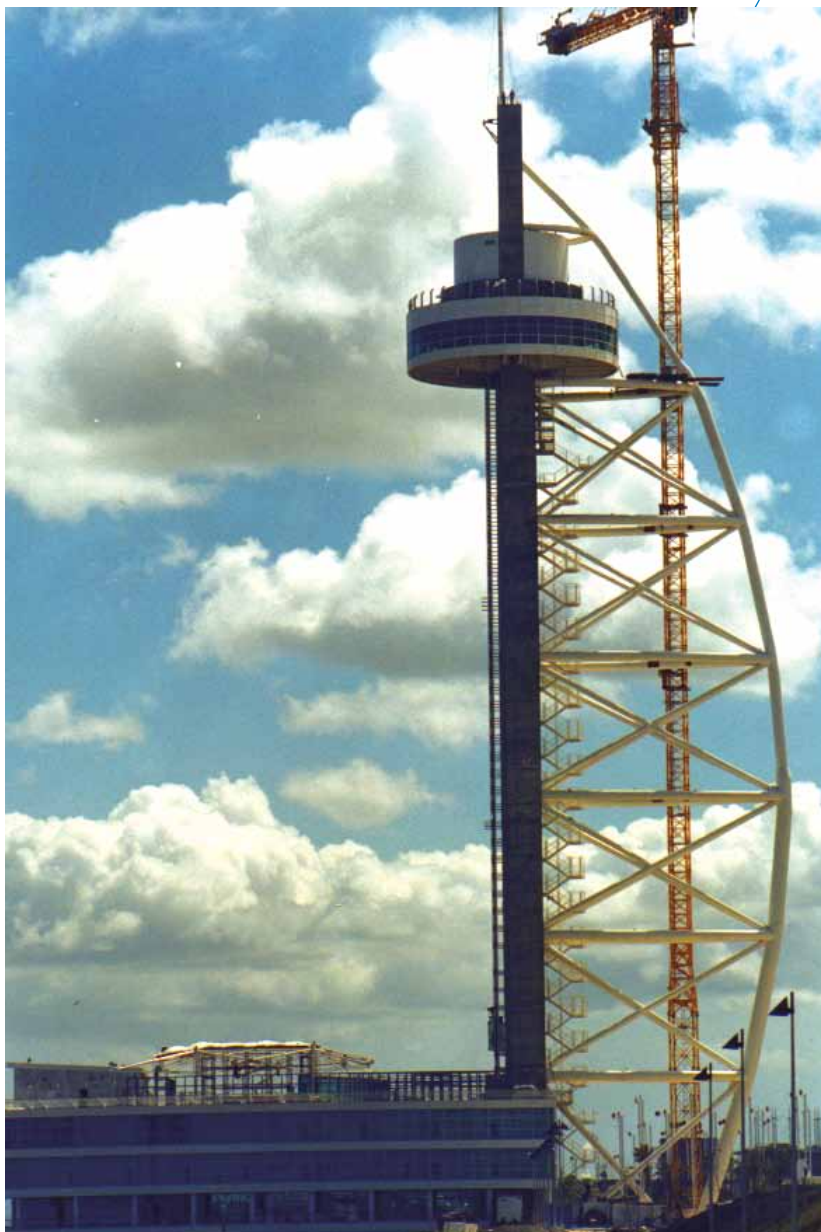
1998 / LISBOA - PORTUGAL Erection of Steel Structures for the Vasco da Gama Panoramic Tower EXPO'98
